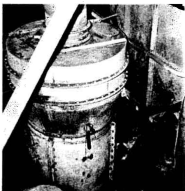
One of two big Raymond Mills grinds raw ore to powder in preparation for the mixing, curing, or finishing which precedes the bagging or bulk shipping. The mill is fed from the hopper at right.
