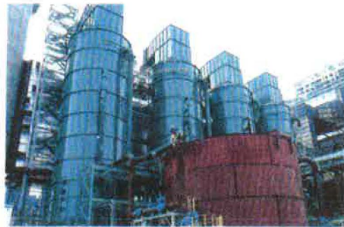
Air pollution-control equipment on all System lignite units helps ensure that air-quality standards are met.
