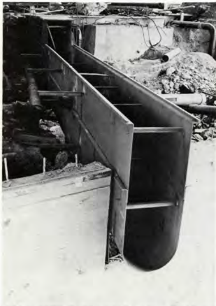
One of the troughs of the chip conveyor during installation. The high pressure nozzles force the shavings through this flume and into the separator. The system has resulted in a considerable savings of time and labor.
