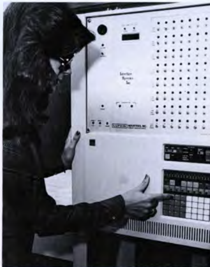
Wanda Camp, plant engineering, looks over LUFKIN's new Energy Management System. The IBM computer, designed especially for monitoring large electrical systems, will save nearly $100,000 a year, paying for itself in only eleven months
