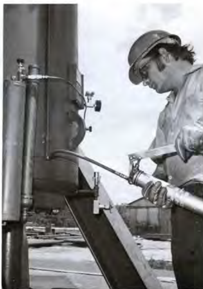
Robert Foley, utility maintenance, shows how to oil pumping unit parts. Robert was part of a crew which put together a pumping unit for photos
