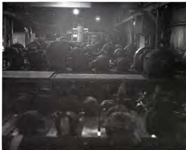
After three months of carrying out a clean-up project, the air compressor building had its material and battery motors tagged, and placed on shelves
