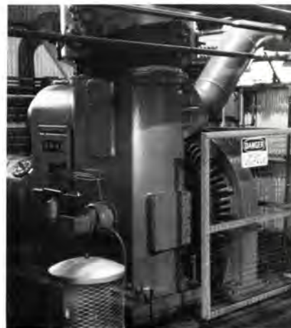
Gene Hargis, foreman, electrical department, believes the men want a clean place to work. Apparently, he is correct because a look at any of the air compressors in the air compressor building reflects a clean, shining surface
