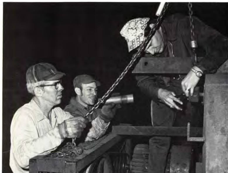
Counter clockwise: Buddy Jones, Mike Kizer, and Jim Bowman, foundry electrician, pull the oven fan to replace belts and hubs in the foundry mold oven
