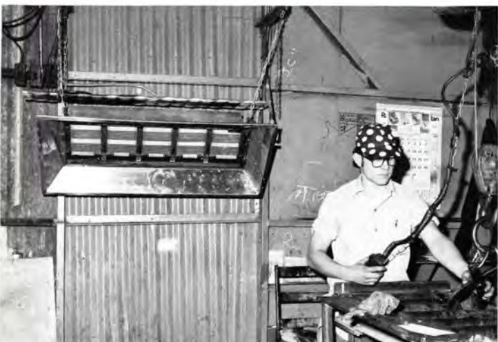
Pot burners, which burn natural gas without thermostats, are being replaced by the larger Dravo heaters with thermostats like these (at top) in the Machine Shop and infrared heaters, like this one (above) in Bobby Colbert's work area. The Dravo and infrared units heat with much less energy than pot heaters
