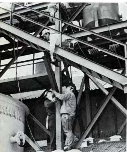
STAIRWAY installed which goes to top of cupola system for problem detection
