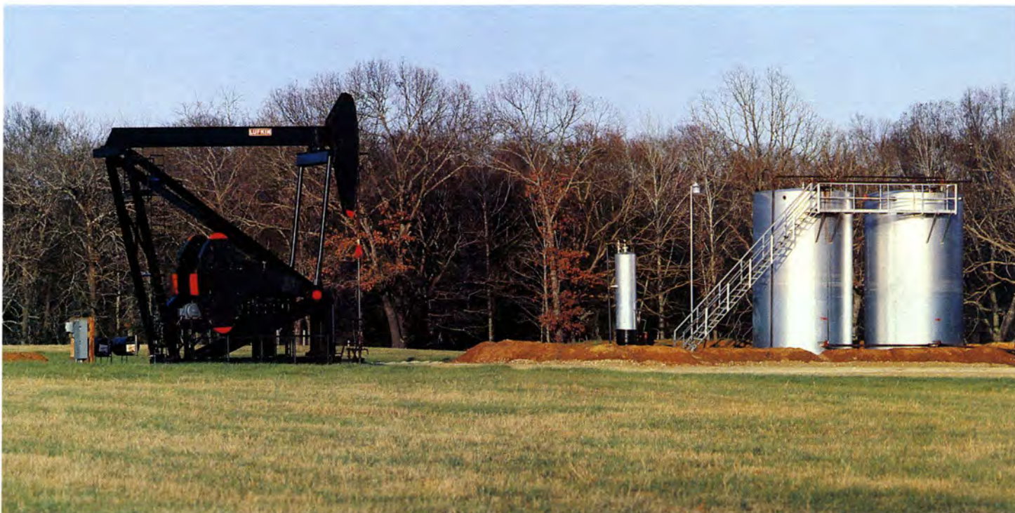
LUFKIN M-640D-365-144, Arcadia Refining Company, Tyler, Texas
