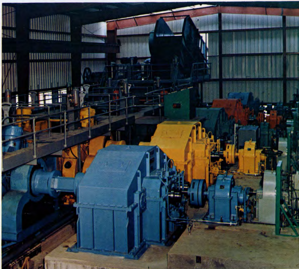
A battery of LUFKIN TC6025H Speed Reducers coupled to LUFKIN TC4431 Speed Reducers driving a sugar mill in New Iberia, Louisiana.
