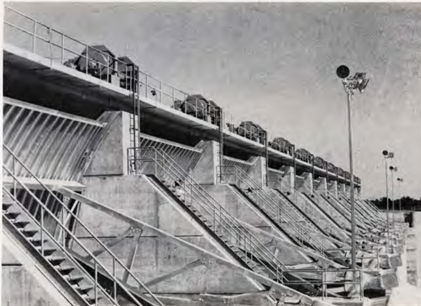
TWENTY-FOUR Lufkin Gear Reducers operate the 12 gates, shown here in a closed position
