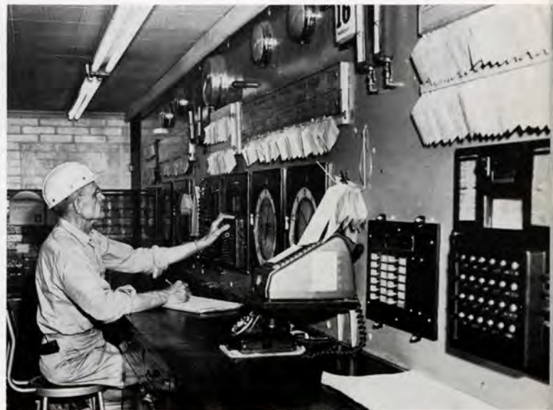
J. E. JIMMERSON checks instrument readings in the central tunnel kiln control room.
