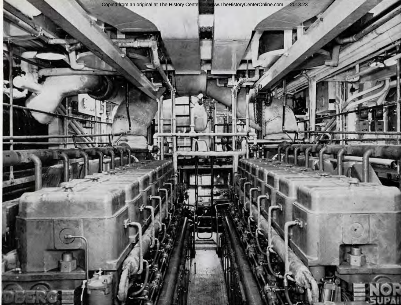
TWO NORDBERG 2500 HP eight-cylinder Supair-thermal diesels aboard the "Henry Foss" replaced
