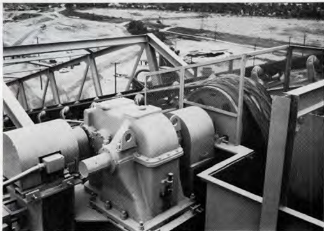
LUFKIN 160D HI-Q Reducer, 25 HP motor, 1200 RPM, 29.4-1 gear ratio, drives the Number Two crushed rock conveyor.
