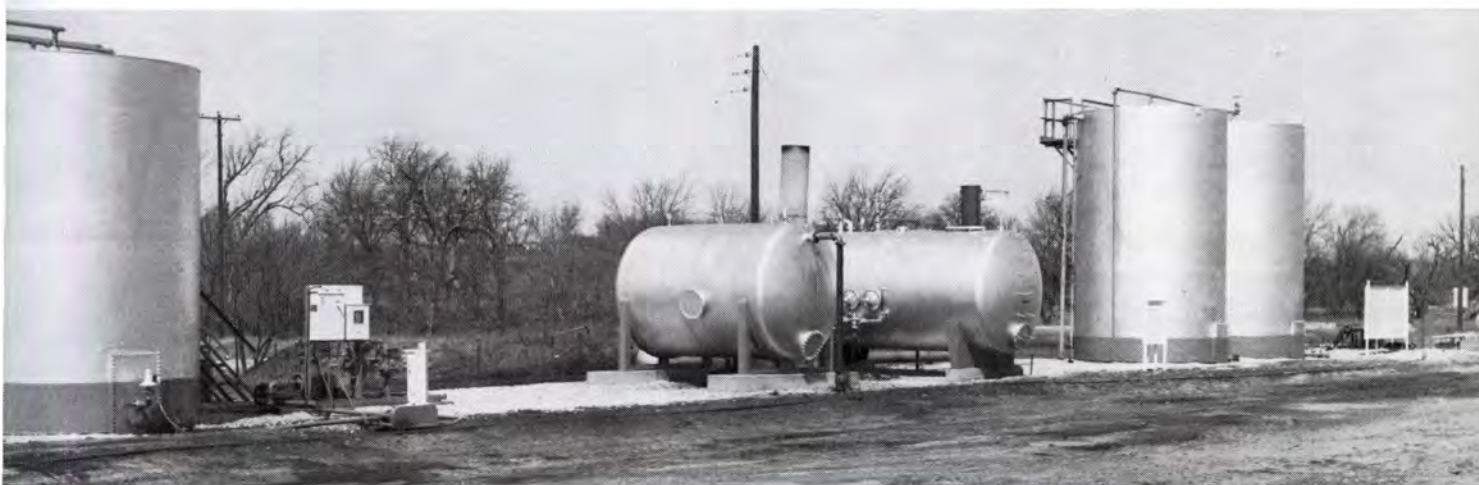
BRUHLMEYER central tank battery. From right to left: test separator on far right, produced water storage tanks; chem-electric treater, and free water knock-out; LACT unit; and discharge storage tanks
