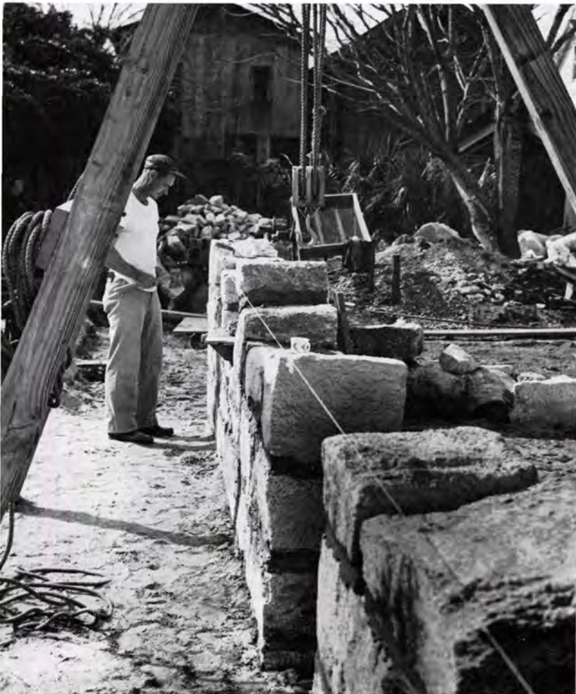
THE first story of a two-story reconstructed Spanish home is under construction in this picture. Workmen painstakingly follow exacting plans to make each home and building authentic
