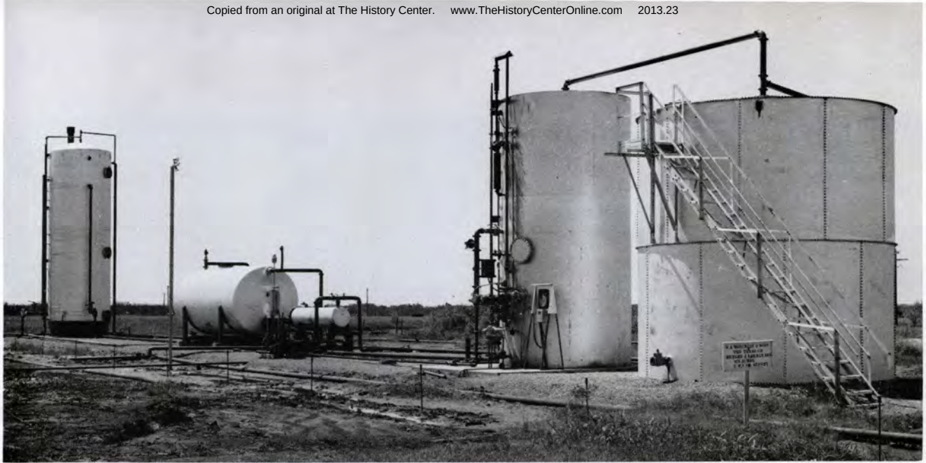
FIGURE #4: Heater-treater, free water knock-out, LACT unit, and storage tank.
