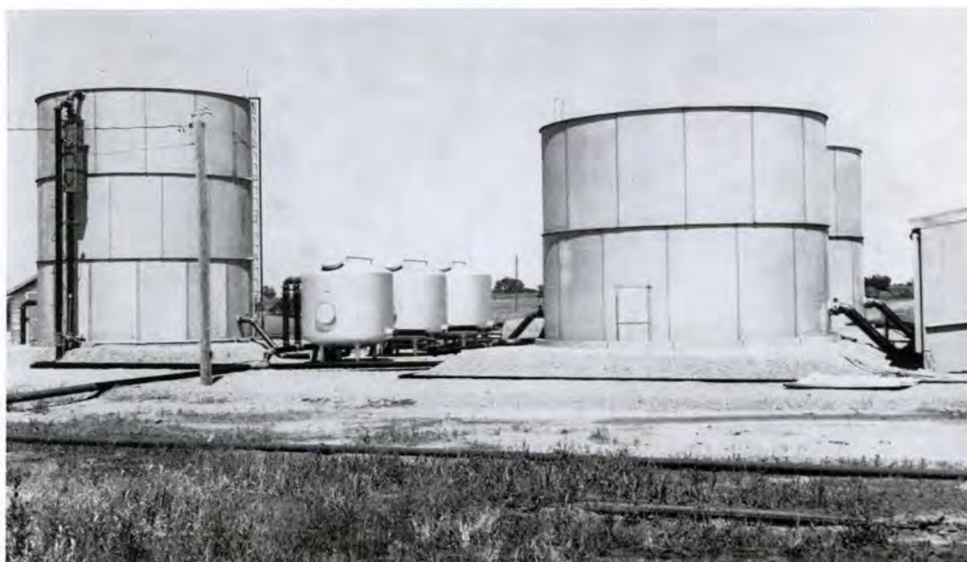
WATER INPUT SYSTEM: Produced water storage tank on left; filters for produced water in the center; and temporary storage tanks for both produced and fresh water on the right. The pump building is on the extreme right.
