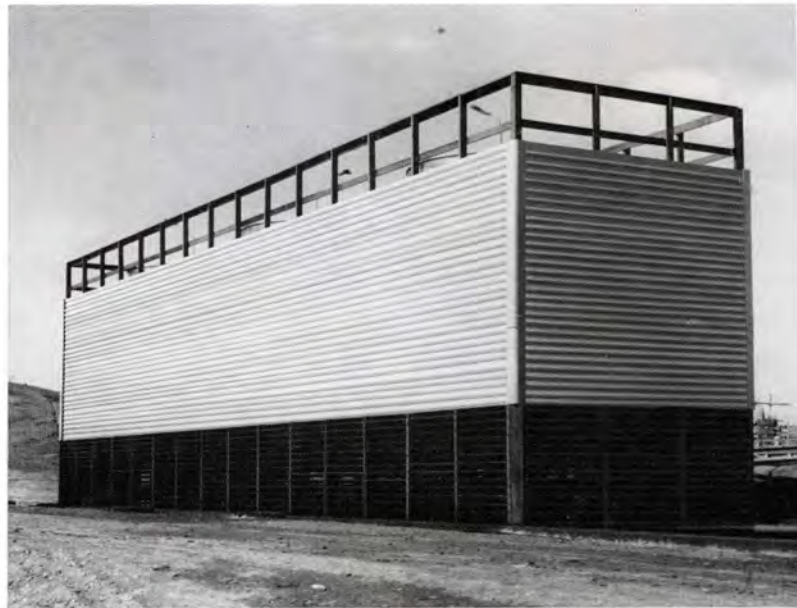
THIS modern, high efficiency induced draft cooling tower at a Southern California oil facility was converted from an atmospheric type tower of twice the size by Fluor Products Company, Santa Rosa, California. Lufkin supplied the three model 50-VB spiral bevel gear speed reducers
