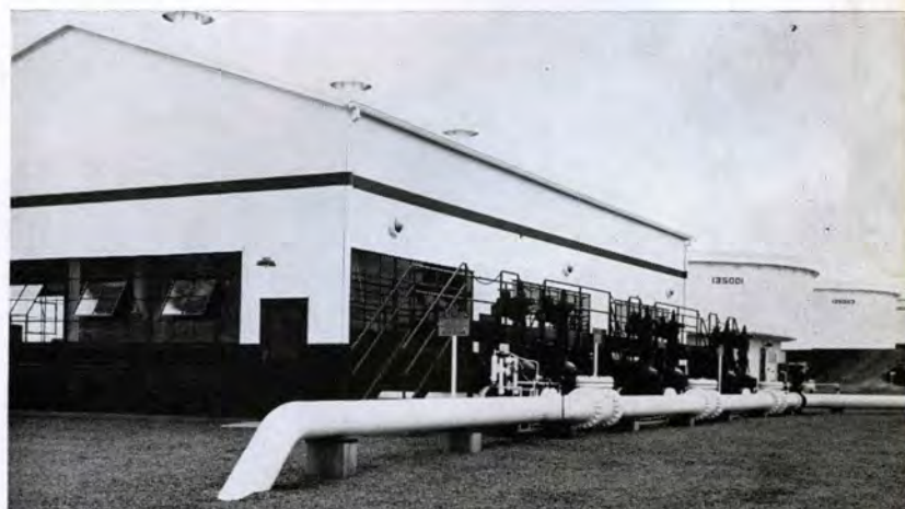
Coalinga Pump Station boosts oil northward to Oleum at 85,000 barrels per day.
