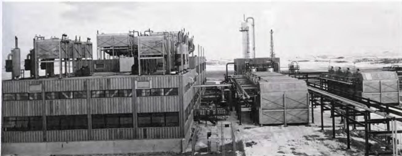
THESE are generator-compressor bldg., first and second stage after-coolers, and third stage gas after-coolers
