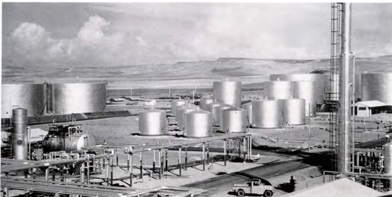
THIS battery of storage tanks at Batman is part of the Turkish Petroleum Refinery, engineered and constructed by Ralph M. Parsons Co., Los Angeles
