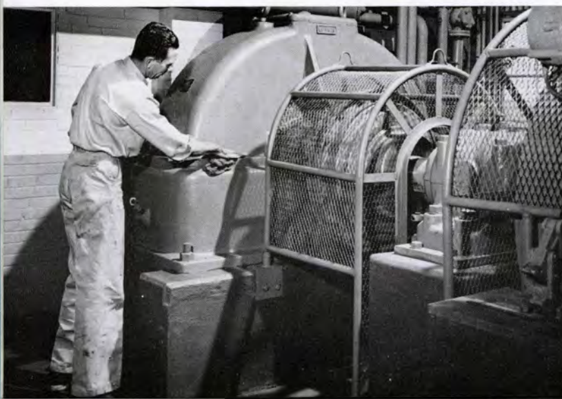
CHIEF Engineer at Gaines Station wipes away dust from increaser. Cooling water piping in background
