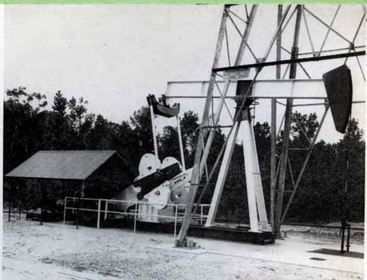
LUFKIN TC-1A-54B unit driven by LUFKIN GSDH engine bolted on extension base. Richardson and Bass, operator, Rapides Parish, Louisiana.
