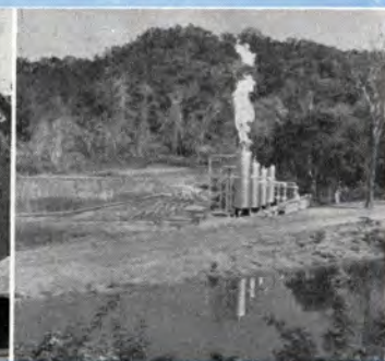
A separator station of the Venezuelan Atlantic Refining Company, Tucupido District, Venezuela.
