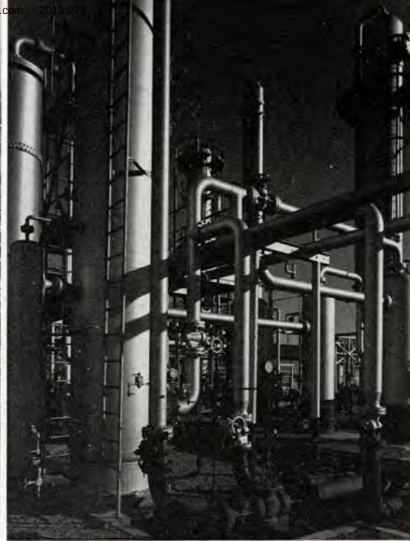
THIS ABSORPTION PLANT operated at Santa Maria by the Union Oil Company extracts carbon dioxide from its crude oil and turns it into commercial dry ice.
