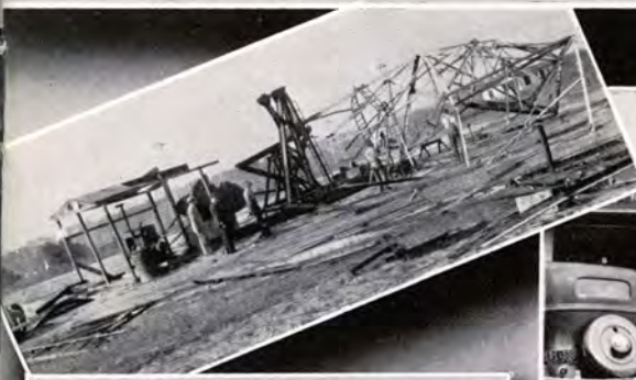
Recent Wind Storm in East Texas. Sutton & Hawkins Oil Co.'s Derrick blew down, knocking off beam—damaging only center of Bearing Caps. No. 31-C Unit—25' plain beam. 15' 3" post.
