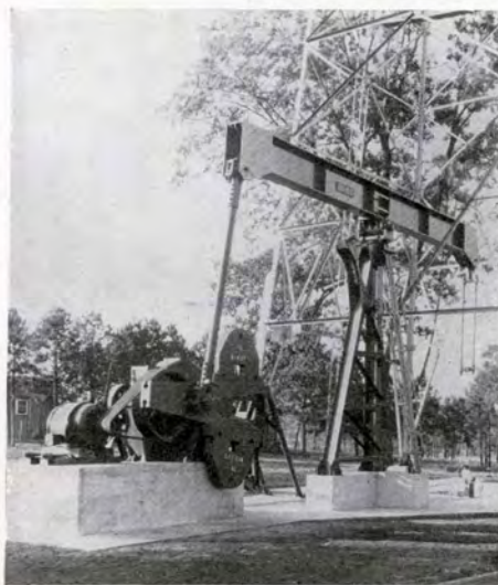
Lufkin No. 58 Herringbone Unit complete with Center-line Beam Assembly and arranged for "Back-side" crank pumping of two extra wells—see details of crank arrangement on opposite page. Lechner & Hubbard, Castleberry Lease.
