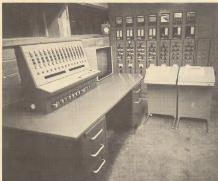
Digester Control Room showing Nokia Autocook operator console in left foreground, television monitor center, two teletype printers, right, and new digester manual control [back-up] panel [digester 6-12] in the rear.
