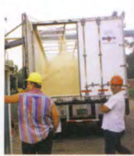
The new outfeed system at Diboll Particleboard loads sander dust into trucks to be hauled away for the production of value-added products currently being researched.
