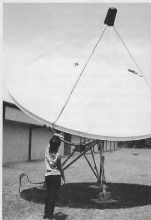
DEBRACCA GOFF looks at the 16-foot satellite dish that is installed behind the school to receive signals for the T-STAR system.
