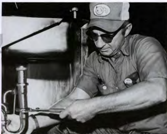
The machinery electrical group also handles all plumbing installations for the Machinery Division. Here, James Hines installs a water fountain in the new industrial gear building.
