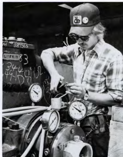
Tim Daniel, a member of the electrical installations crew, wires an industrial gear unit.
