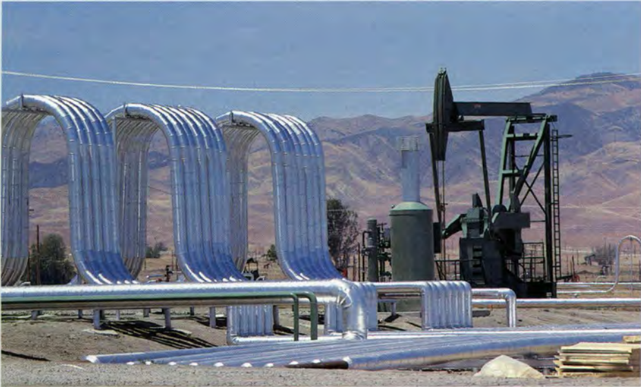
LUFKIN M-228D-173-100 Unit, Chevron USA, Fresno County, California.
