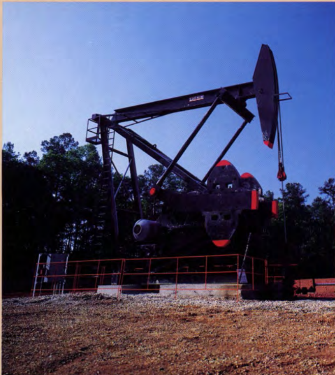
LUFKIN M-912D-365-168 Unit, Stone Petroleum Corporation, Greensburg, Louisiana.
