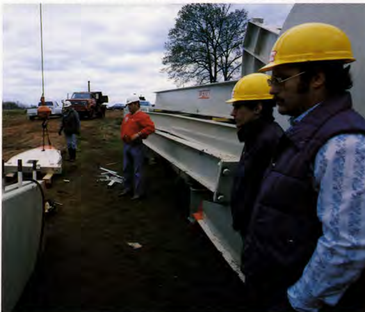
Braving a cold morning in an East Texas oil field near Quitman, Texas, LUFKIN employees, Mike Whitten and Vernon Speicher, Jr., watch as crews begin unloading a 70,000-pound M-912D-305-192 pumping unit.
