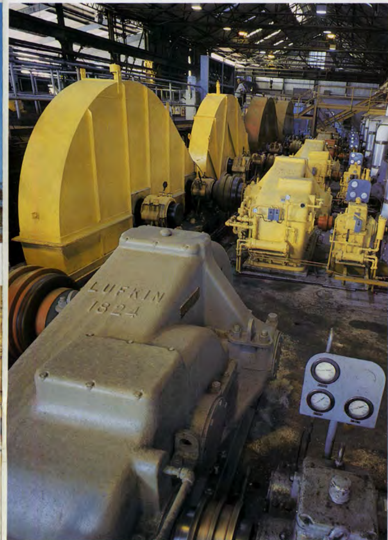
LUFKIN N1204C Gear Reducer with LUFKIN D1824 Double Reduction Gears drive a spur gear final-drive and Fulton three-roll sugar mill in a Florida sugar factory
