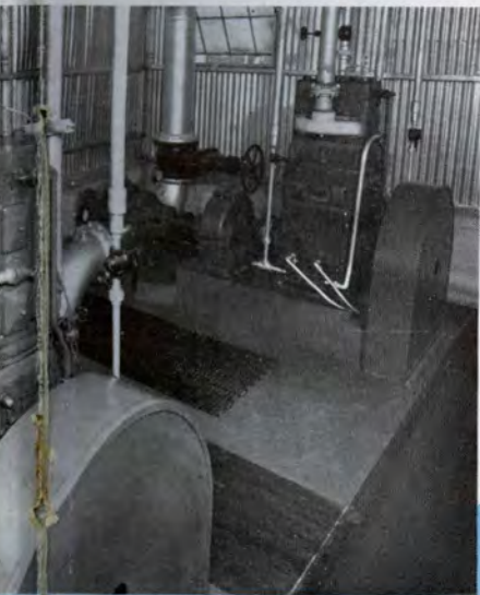
1. Lufkin GSD with Lufkin 5105 Speed Incentrifugal water pump, pumping against a 45-foot head; Warren Petro-20; Fairbanks, Texas.
