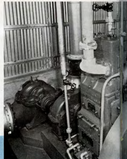
2. Dual installation of Lufkin D creaser driving a 12-inch centrifugal pump discharging 3800 gallons per minute against a 40-foot head. Lufkin Petroleum Co., Plant 2 Fairport, Oklahoma.
