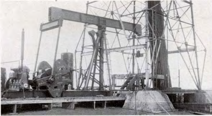
INDIAN TERRITORY ILLUMINATING OIL COMPANY — OKLAHOMA STATE NO. 9 Lufkin completely equipped, consisting of: No. T.C. 1A-56 Unit with No. 1028-C walking beam assembly, and three cylinder National Transit 40 H.P. engine. Installation is one of many similar ones in the Oklahoma City field.
